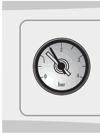
Sealed System pressure when boiler is operating
